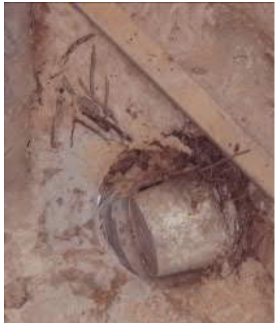
Figure 2: Check for large debris and standing water above the fiberglass inserts
