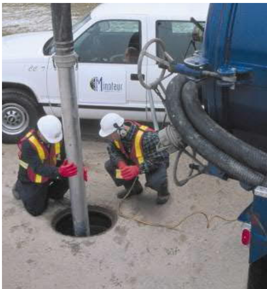
Figure 35: Vacuum truck line, at-grade
