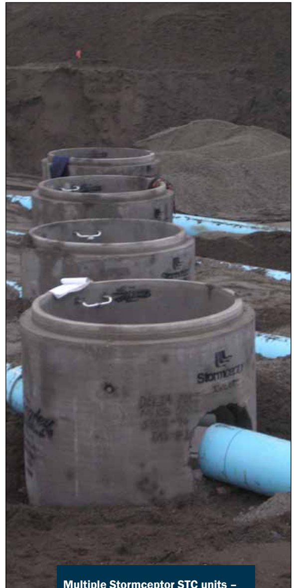
Multiple Stormceptor STC units – provides stormwater treatment and spill capture at the Delta Port in Vancouver, British Columbia, Canada
