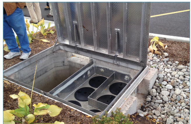
A Jellyfish Filter pretreats a bioretention/bioswale system at a commercial site in Ontario, Canada.
