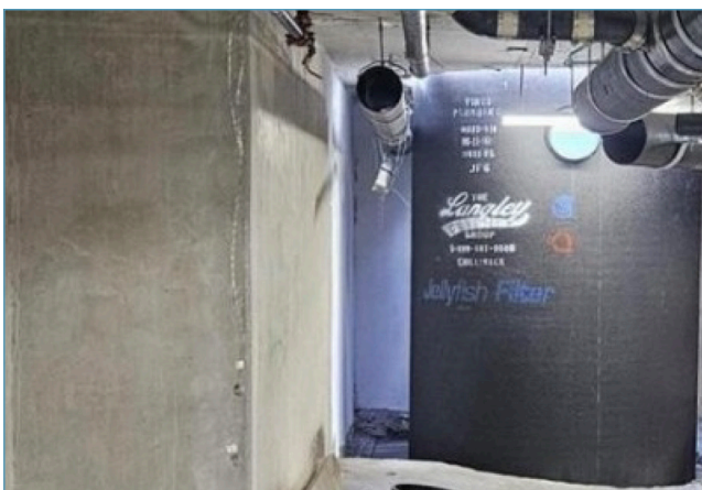
A Jellyfish Filter provides treatment to high rise tower before detention storage or water re-use in British Columbia, Canada.
