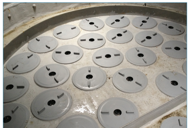
A Jellyfish Filter provides treatment at an industrial park in Quebec, Canada.
