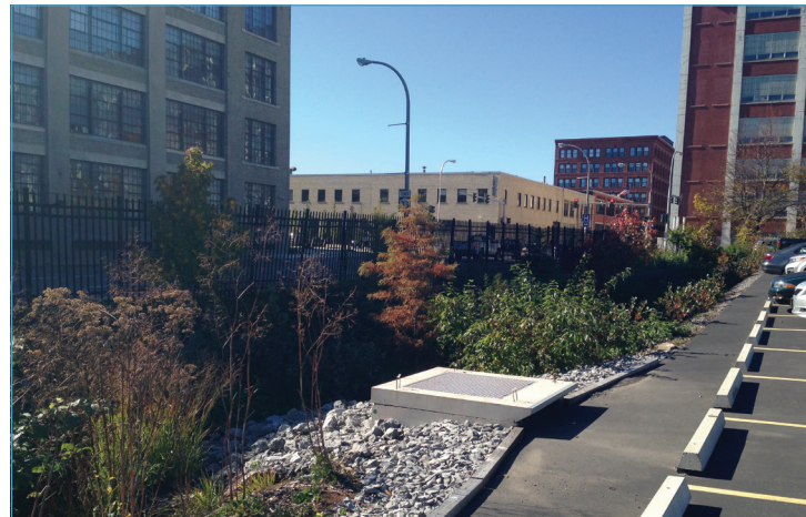
A Jellyfish Filter Curb Inlet pretreats runoff entering a bioretention system.
